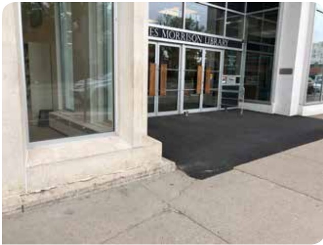
Cracked and crumbling entrance
