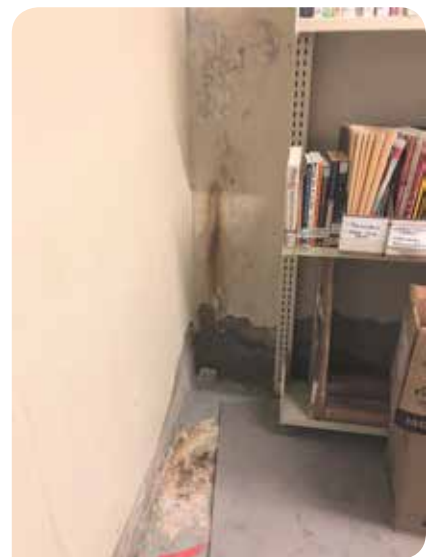
Water damaged and crumbling foundation
