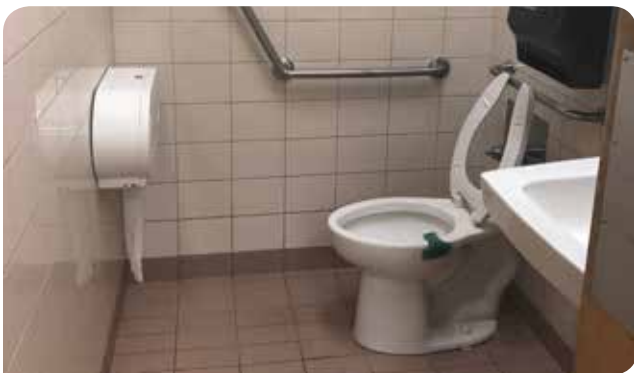
Only one washroom large enough to be accessible
