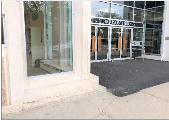
▲ Cracked and crumbling entrance. Repairs addressed safety issues.
