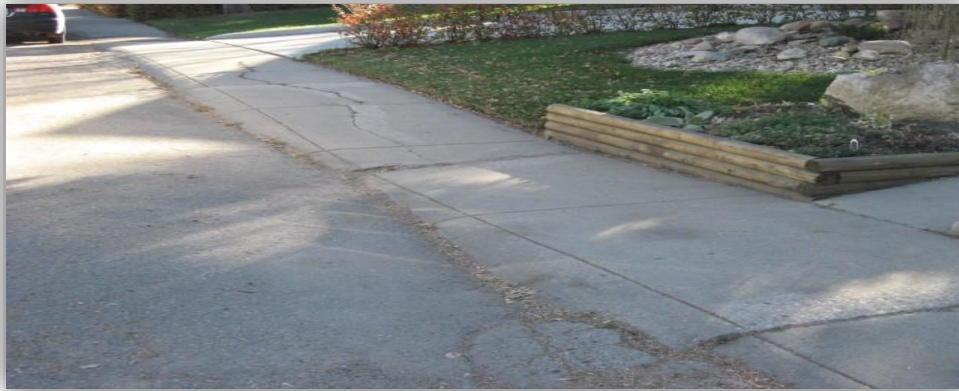
Utility Settlement – Mud Jack or Replacement
