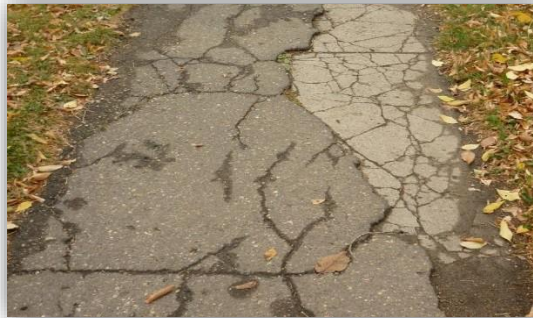
Poor Condition Asphalt Overlay - Replacement
