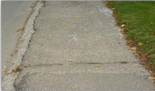
Good Condition Asphalt Overlay Curb Deteriorated - Replacement
