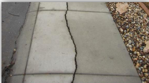
Repair - Crack Fill
