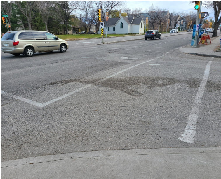
Photo 3 Pavement and Paint Condition
