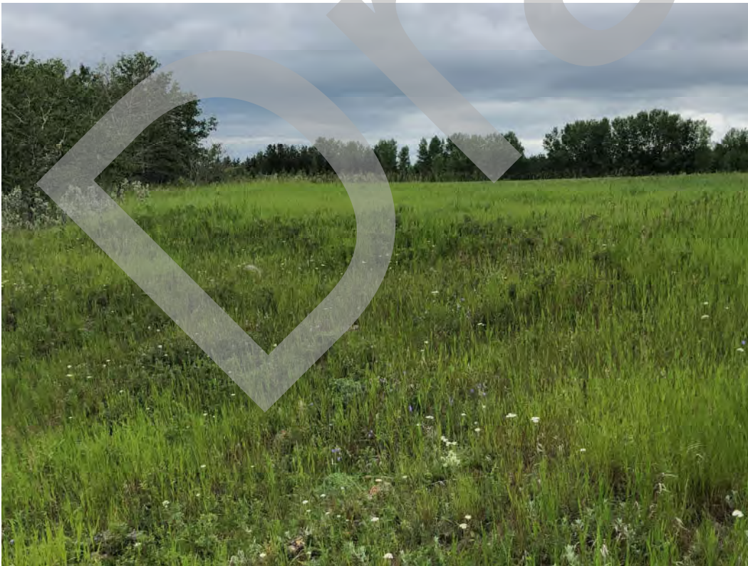
Photo 18 – Middle of East Riverbank – Looking northeast at older debris slide head scarp (at Field Site 3 of 3D Mapping Figures).
