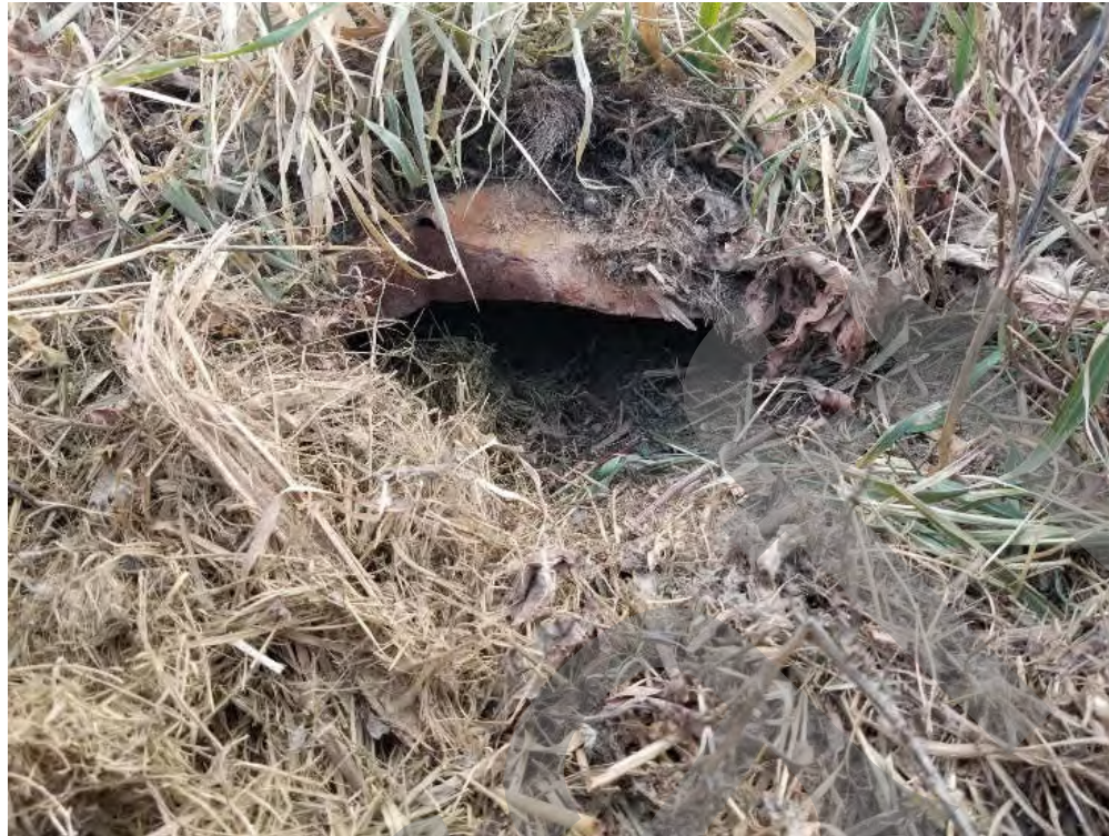
Figure 5.26: Common example of plugged culvert (located in Catchment NN along Range Road 3044, approximately 300 m north of the preferred Freeway alignment)
