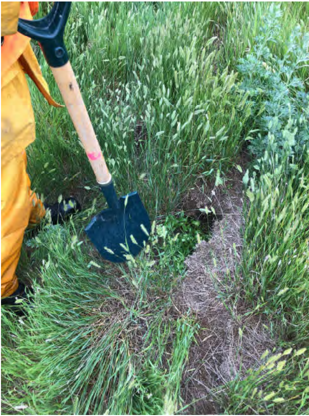
Photo 23 – North side of West Riverbank – Tension crack indicated by small holes - one visible near shovel tip (at Field Site 9 of 3D Mapping Figures).
