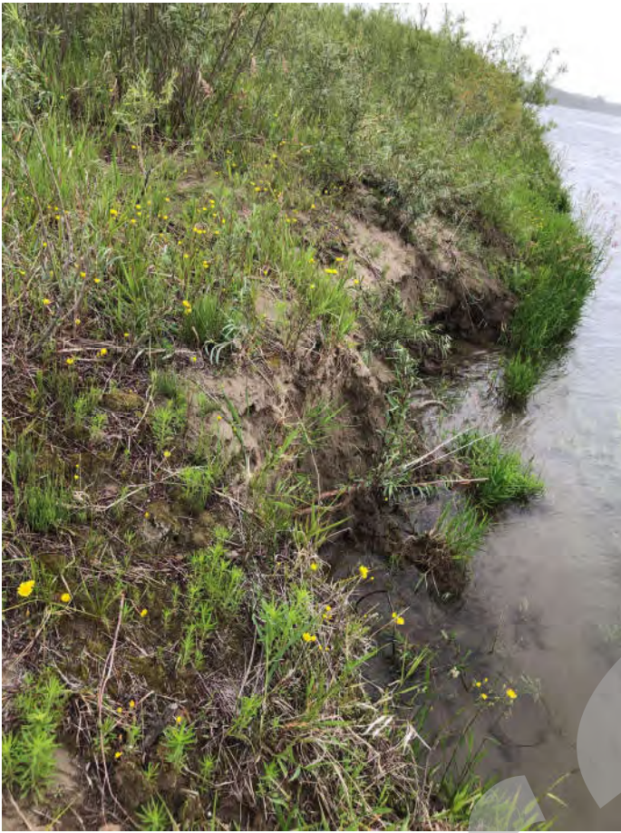
Photo 5- South side of West Riverbank – Looking northeast at riverbank erosion (from Field Site 12 of 3D Mapping Figures).
