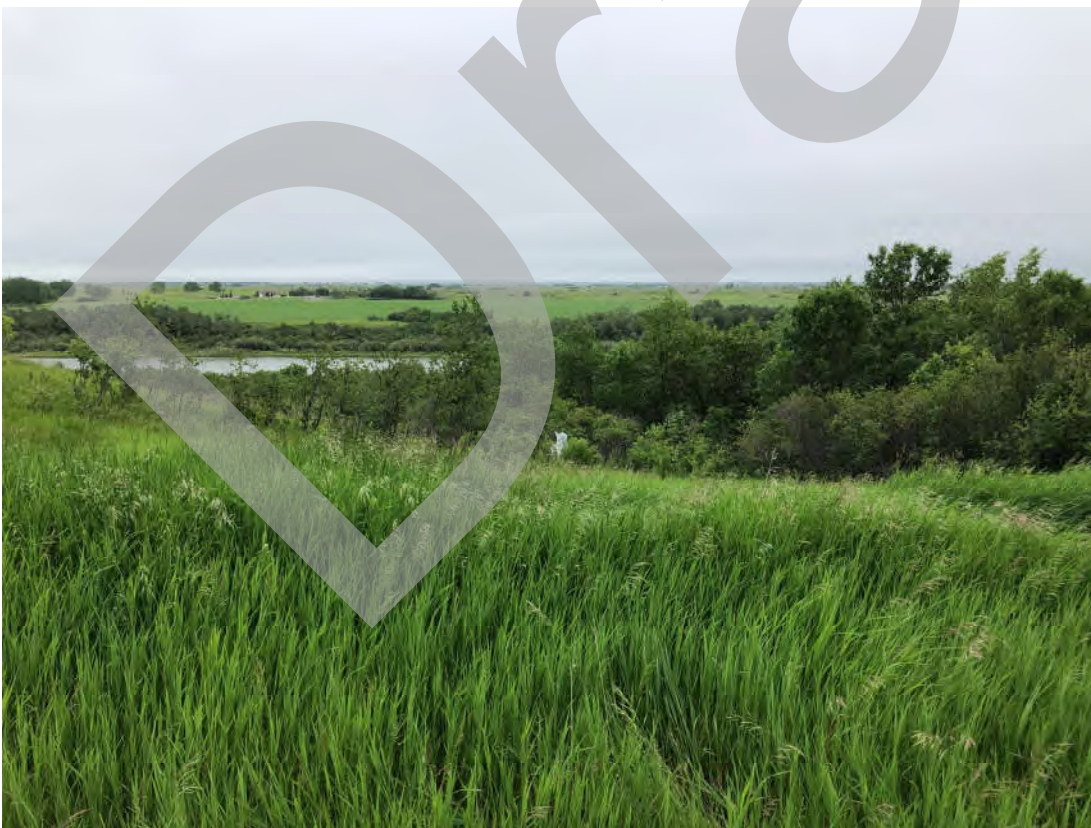
Photo 12 – South side of West Riverbank - Looking southeast at head scarp of small recent debris slide (at Field Site 13 of 3D Mapping Figures).
