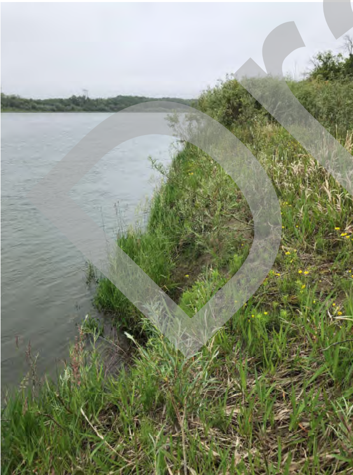
Photo 4 - South side of West Riverbank – Looking southwest at riverbank erosion (from Field Site 12 of 3D Mapping Figures).
