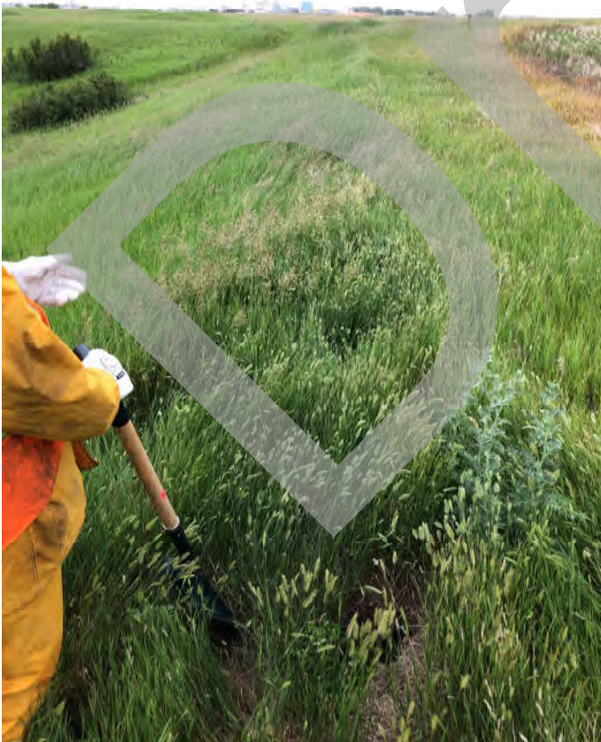
Photo 22 – North side of West Riverbank – Tension crack indicated by change in grass colour (at Field Site 9 of 3D Mapping Figures).
