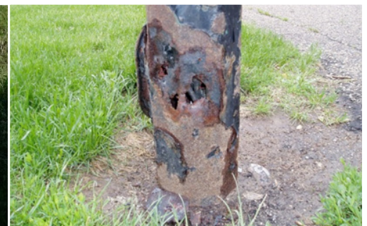
Street Light Pole in Poor Condition
