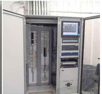
Substation Control Cabinet
