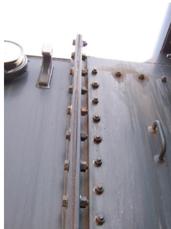
Substation Transformer Oil Leak (1st Ave)
