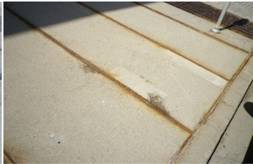
Network Vault Roof in Poor Condition
