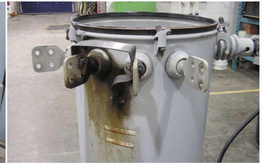
Leaking Overhead Distribution Transformer
