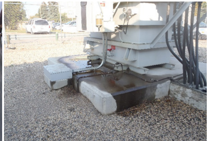
Substation Transformer Oil Leak (College Park)
