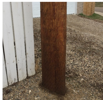
Wood Distribution Pole - New
