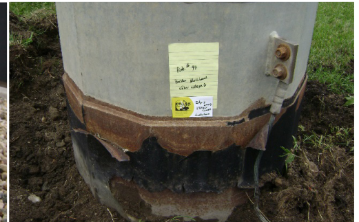
Transmission Tower Base in Poor Condition
