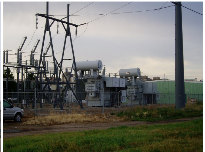
138 kV Transmission Entering Bulk Power Substation
