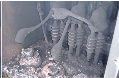
Switchgear Failure from Contamination
