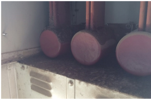
Dirt and Contamination Inside Switchgear
