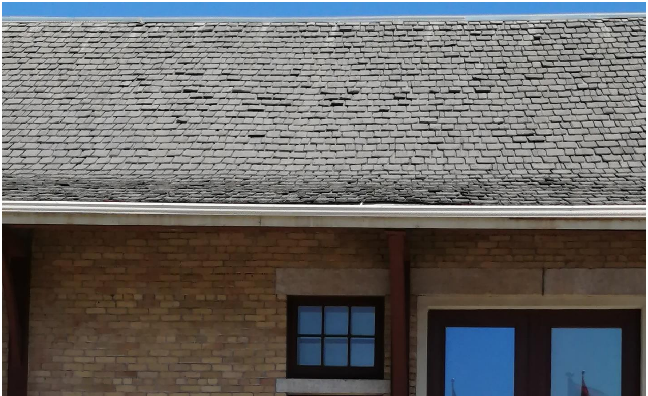
Shingles lifting and splitting
