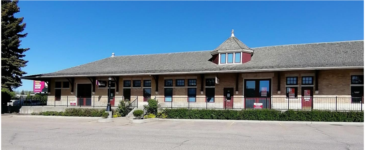
Shingle damage along lower roof section
