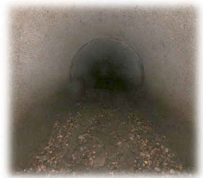
Figure 7: Image of Sediment within Storm Sewer Pipe
