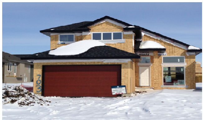
A secondary suite is being constructed in this new home in the Stonebridge neighbourhood.
