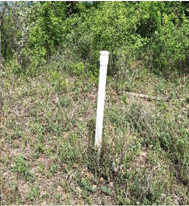
Fig. 3: Well with no protective casing
