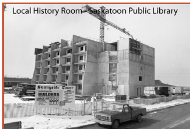
Sunnyside Tower under construction on Hilliard Street West and St. Henry Avenue.
